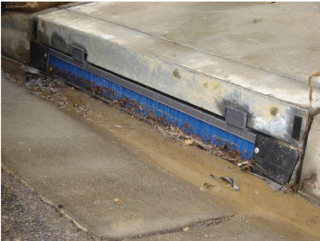
Figure 13: Stormwater Best Management Practice (BMP)
