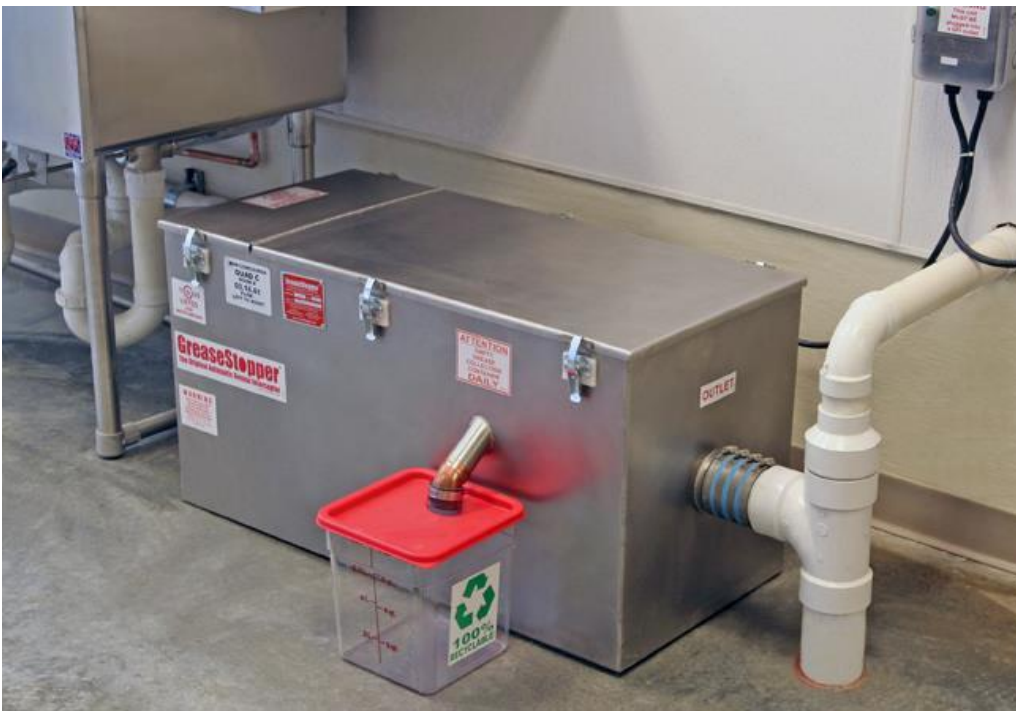
Figure 11: Grease Removal Device (GRD)
